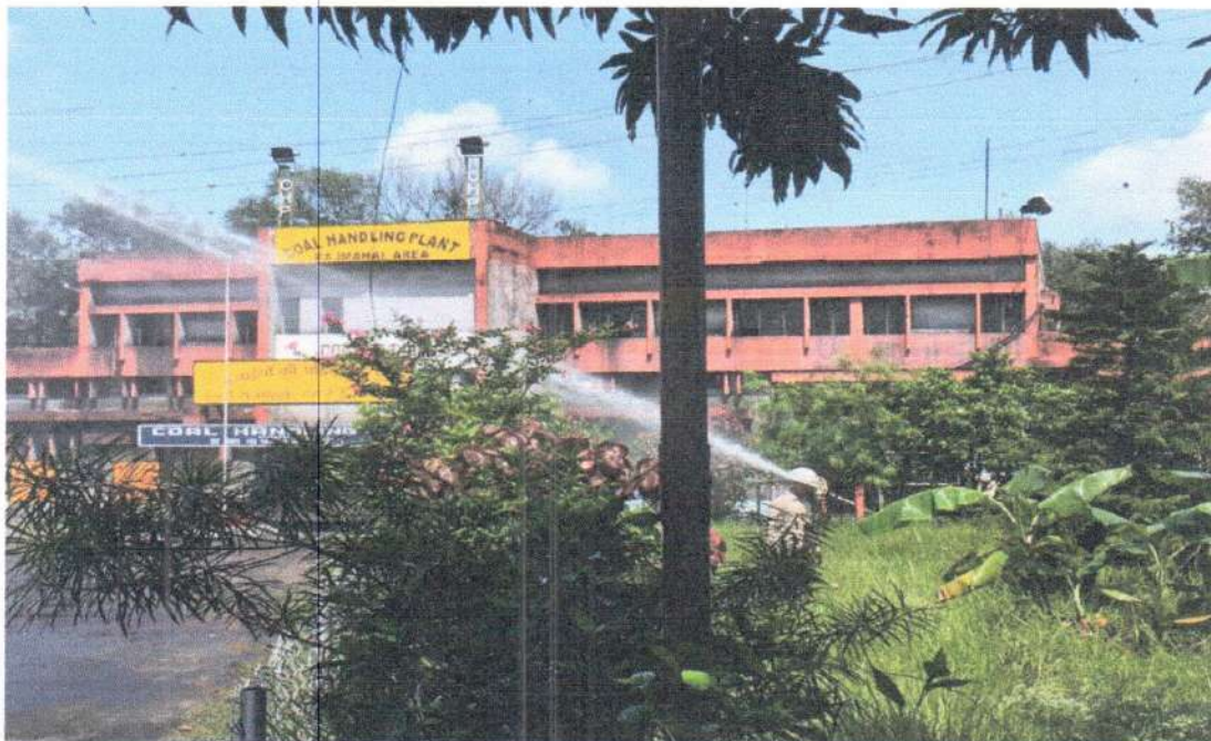
Fixed type water sprinkler at CHP for dust suppression.
