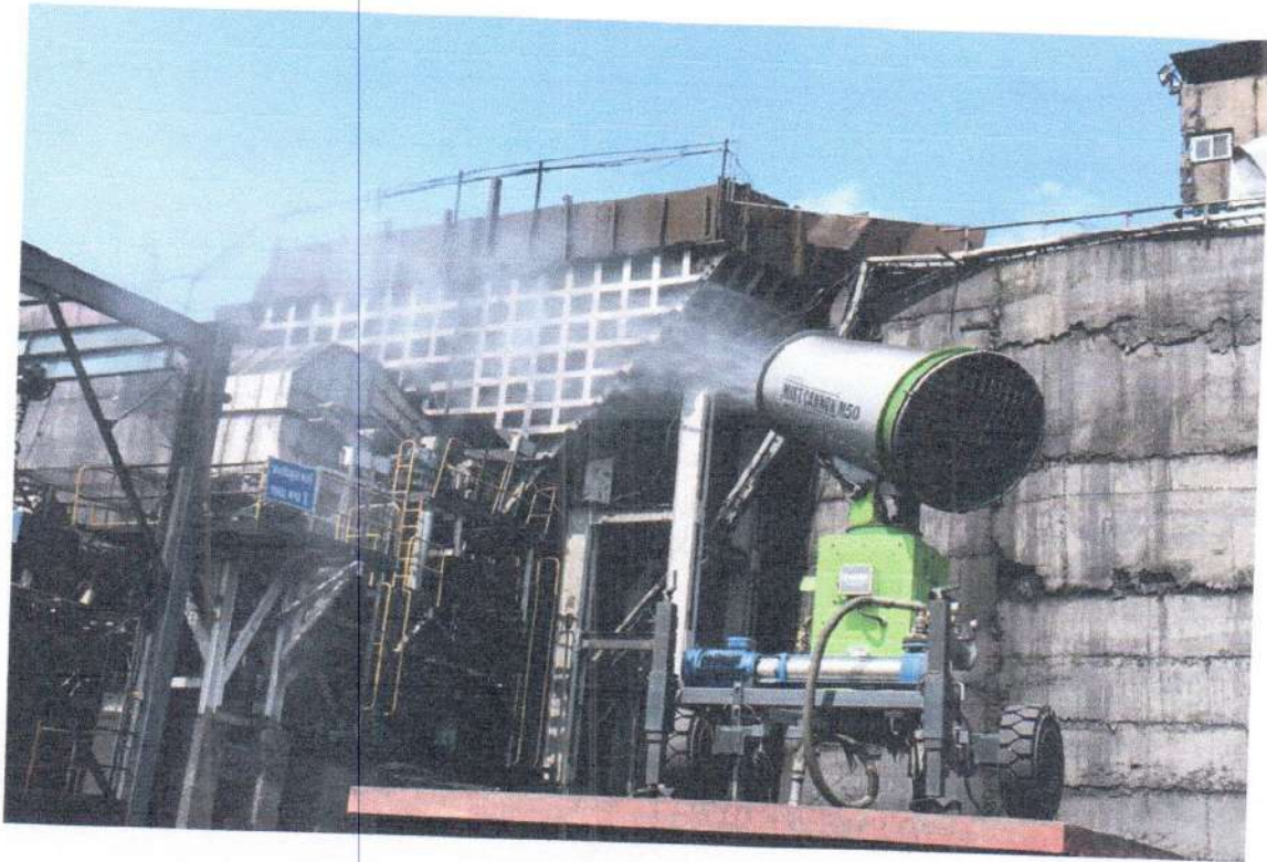
Mist Gun (02 nos.) at CHP for efficient dust suppression.
