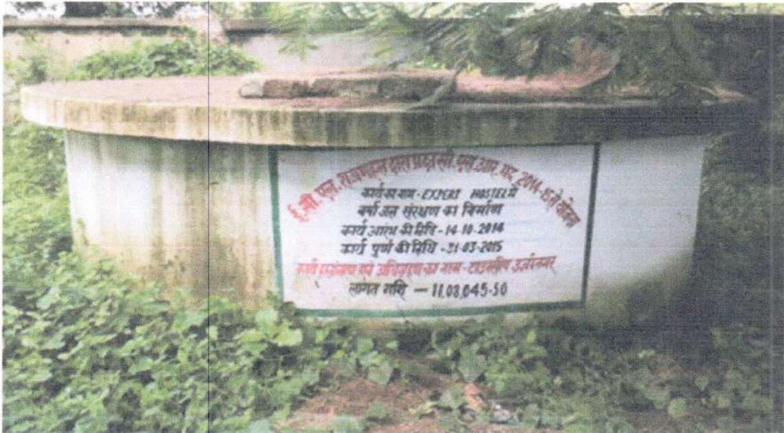
Rain Water Harvesting System (02 nos.) At Rajmahal House (Expert Hostel).
