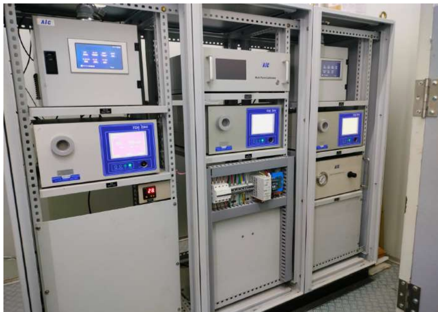
01 no. CAAQMS installed in the cluster.
