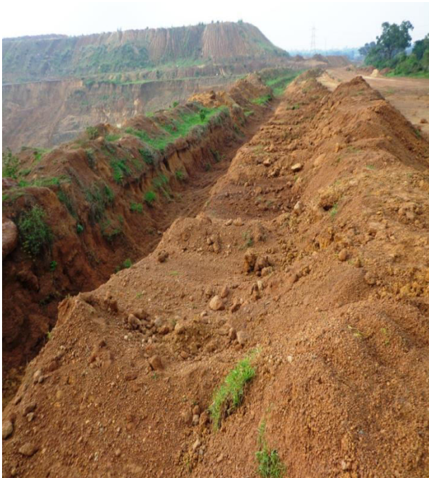
Plate-3: Garland drain around the mine pit of Sonapur- Bazari OCP
