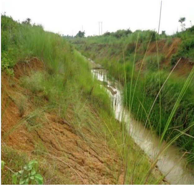
Plate-1: Diverted Tumni nallah bunds not protected with bio-engineering measures
