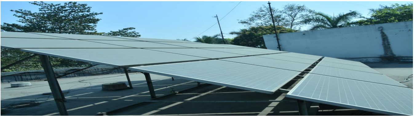
SOLAR PANEL AT SODEPUR AREA VOACTIONAL TRAINING CENTER
