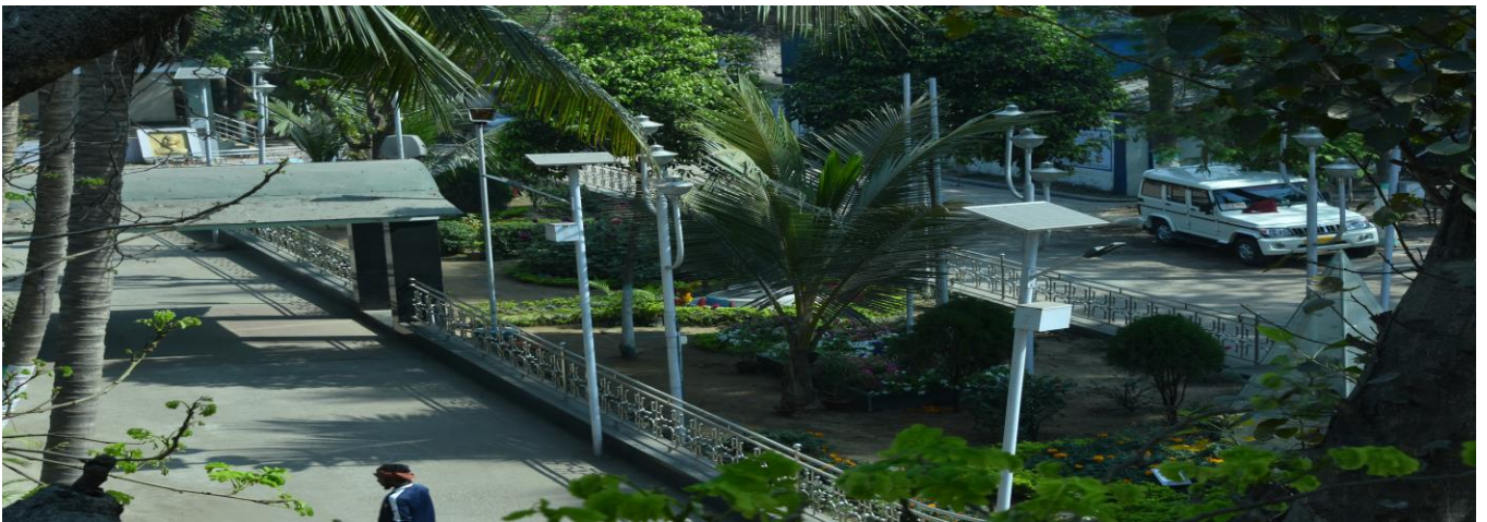
SOLAR LIGHTS AT SODEPUR AREA OFFICE
