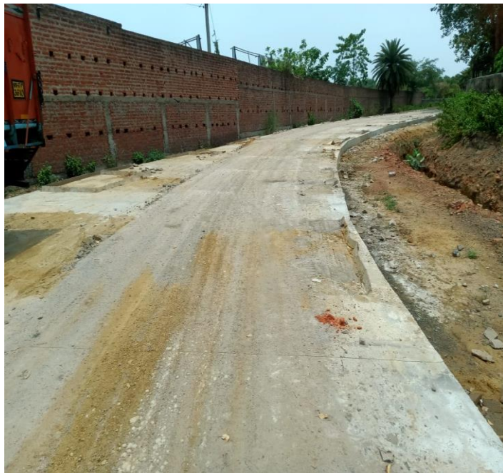
250 mts. approx.. Coal Transporting Road has been constructed from Patmohana Coal Depot
