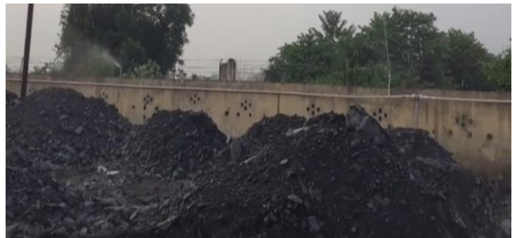
Fixed Water Sprinkling System at Mithani Coal Depot.
