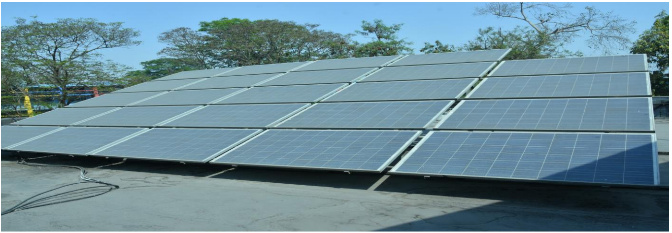
SOLAR PANEL AT SODEPUR ARE OFFICE
