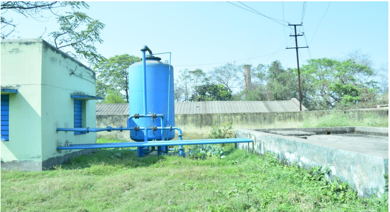
PRESSURE FILTER AT MITHANI COLLIERY
