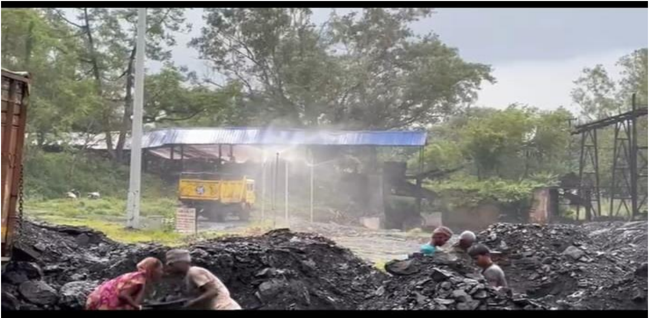
FIXED WATER SPRINKLING SYSTEM AT CHINAKURI RAILWAY SIDING
