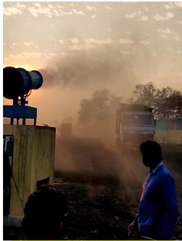
Picture 1: Mist Canon 01at JK Nagar Railway Siding
