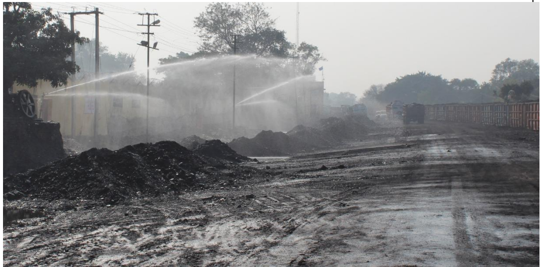
Fixed Type Water Sprinklers at JK Nagar Railway Siding
