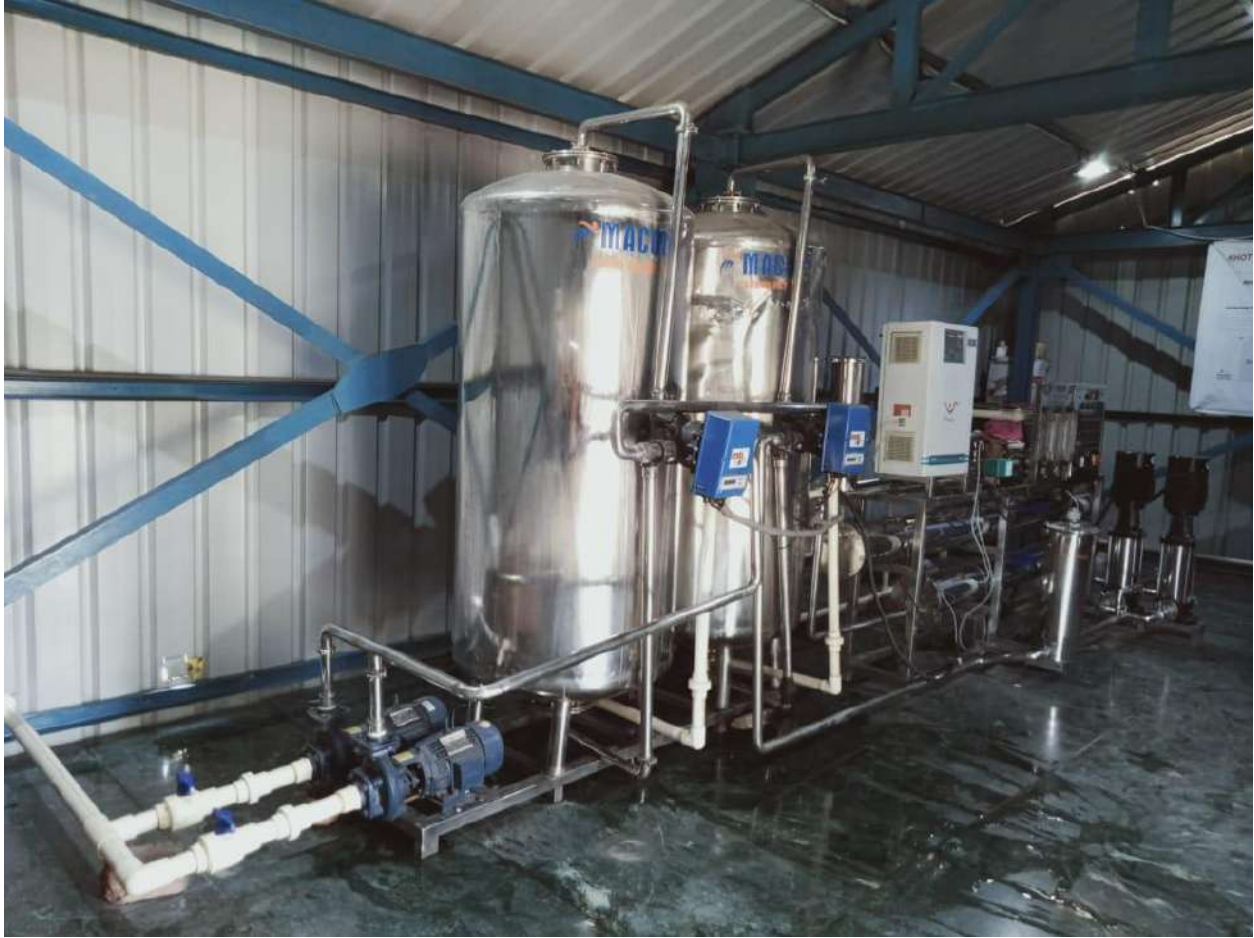
Photograph of RO filtration plant Set up at Khottadih UG
