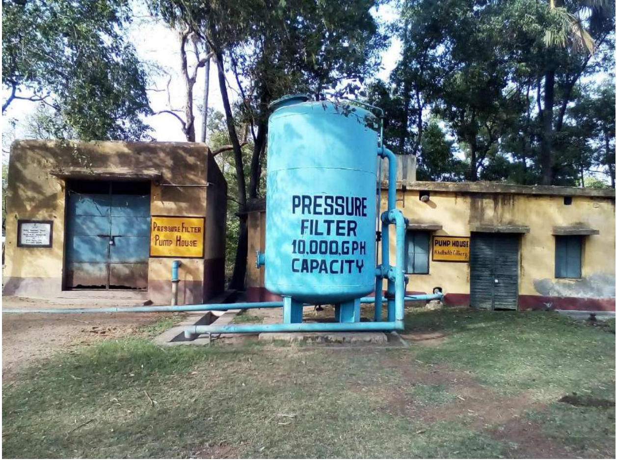
Photograph of Pressure filter installed at Khottadih colony for treatment of mine water.
