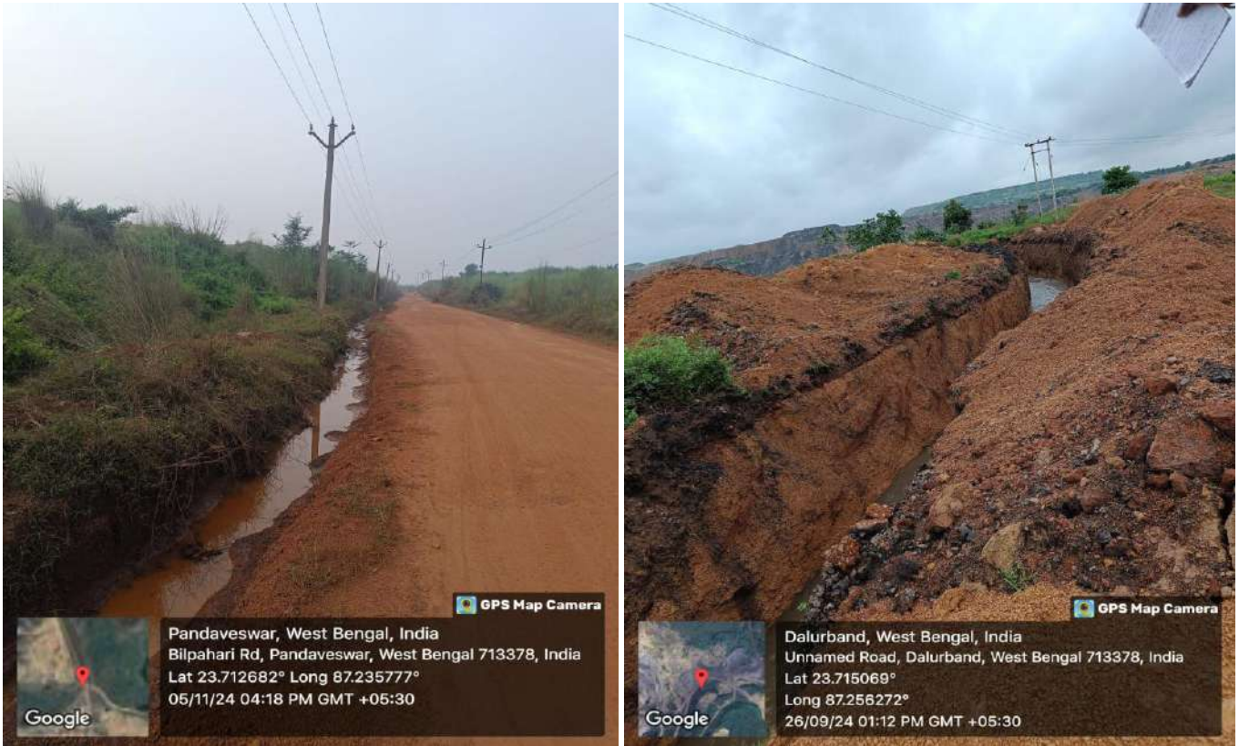
Photograph of garland drain constructed at Khottadih OCP and Dalurband OCP mine
