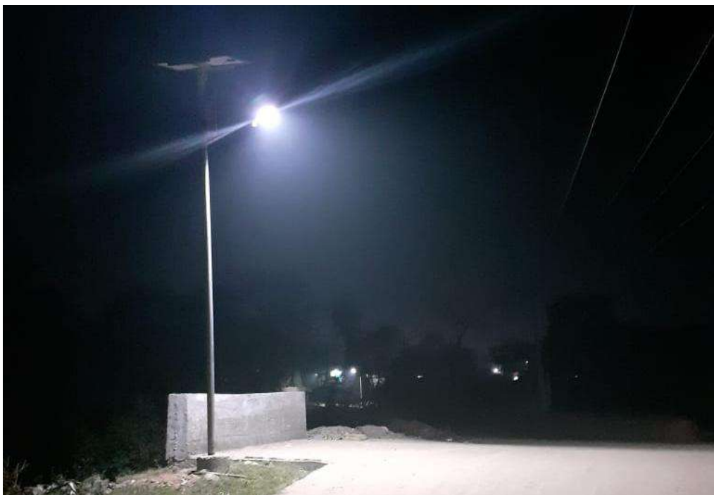
Photograph of Solar street light installed at Baidyanathpur village under CSR scheme of ECL
