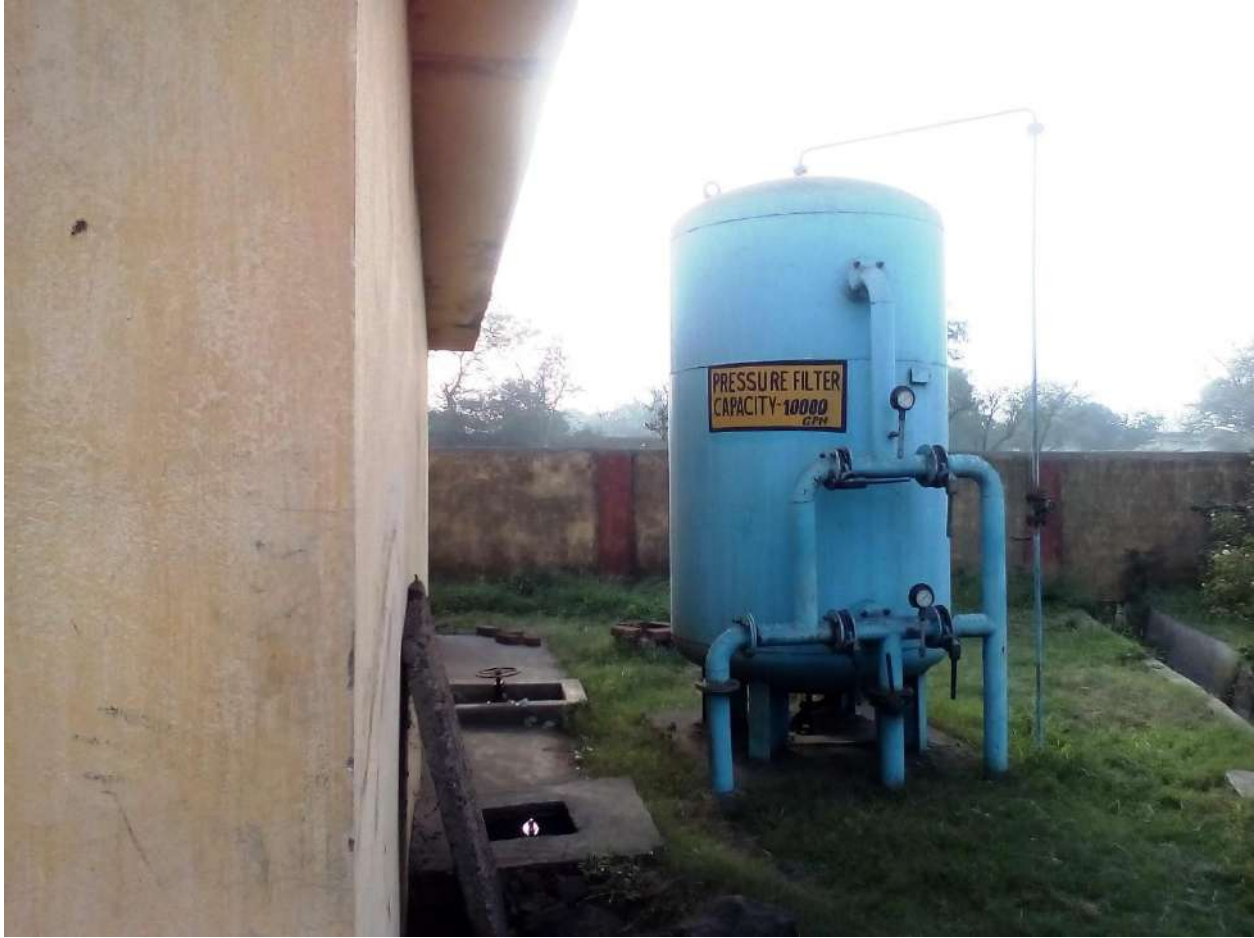
Photograph of pressure filter installed at Dalurband for treatment of mine water
