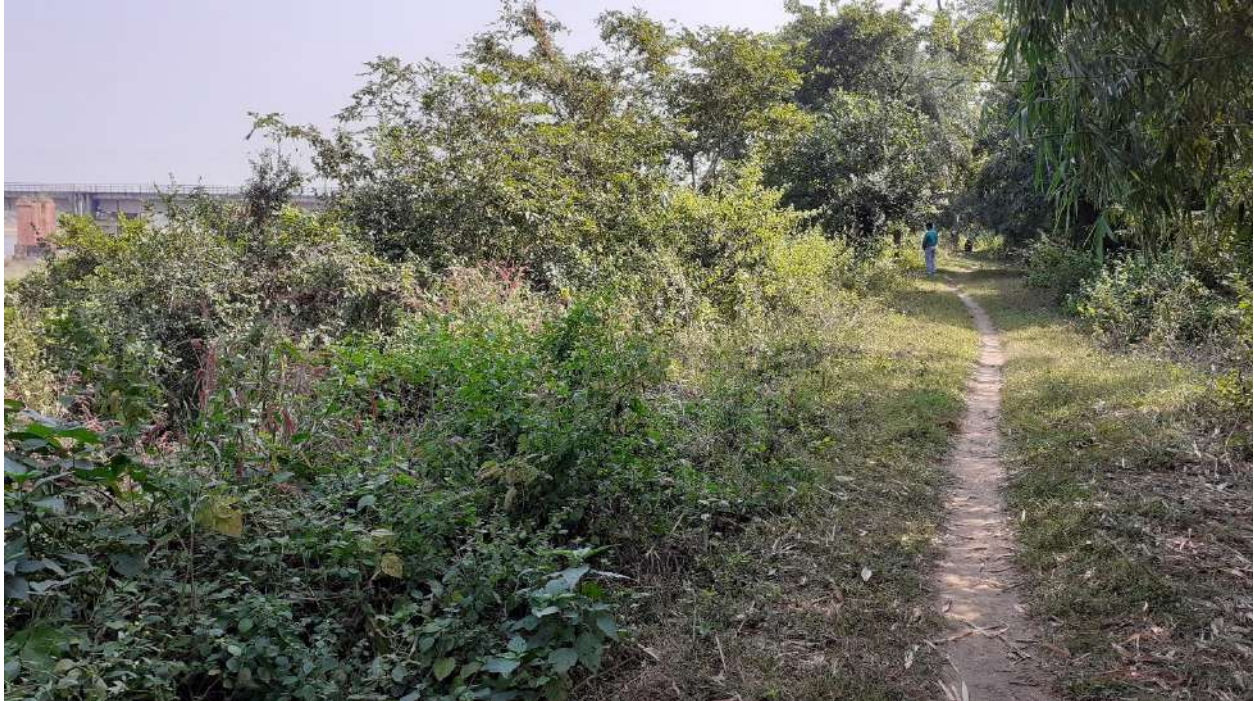
Photograph of embankment constructed and stabilized with plantation along Ajay River nearby Pandaveswar UG mine.
